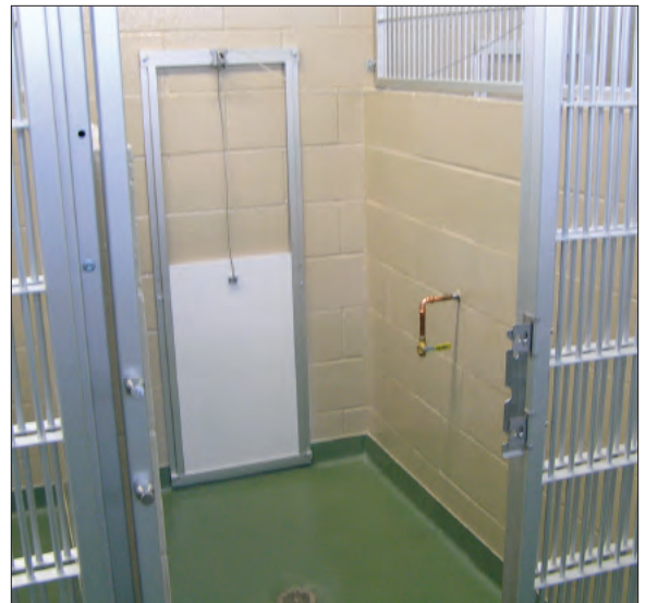
Dogs have their own 4- by 6-foot indoor kennels attached to 4- by 12-foot outdoor kennels. The system used at Stone Mountain Pet Lodge was ICO Glaze epoxy coating system on the block walls, ICO Quartz 120 DB epoxy system on the floors and ICO Quartz Cove providing a seamless transition between the wall and floor.
